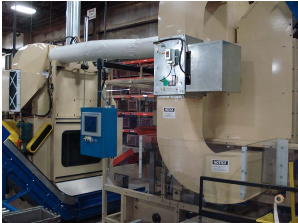
This is a better view of the pre-heat tumbler. It uses the same mesh belt as the spray tumbler. The heated air passes through with the parts tumbling or stationary. Air temperature through the unit is controlled by a thermocouple and the part temperature is controlled by the amount of time spent in the unit.
